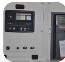
Control Panel & MCB
